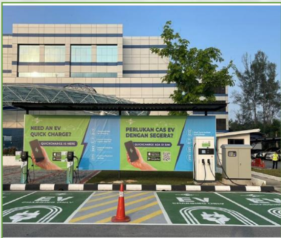
EV Charging in KHTP Business Centre
